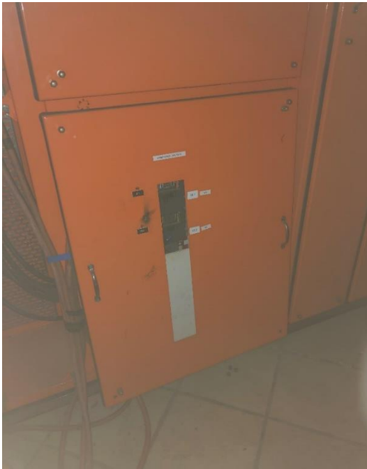
Generator cables run under the front panel. Noting the cable zone to the left of the MSB that should have been utilised.
