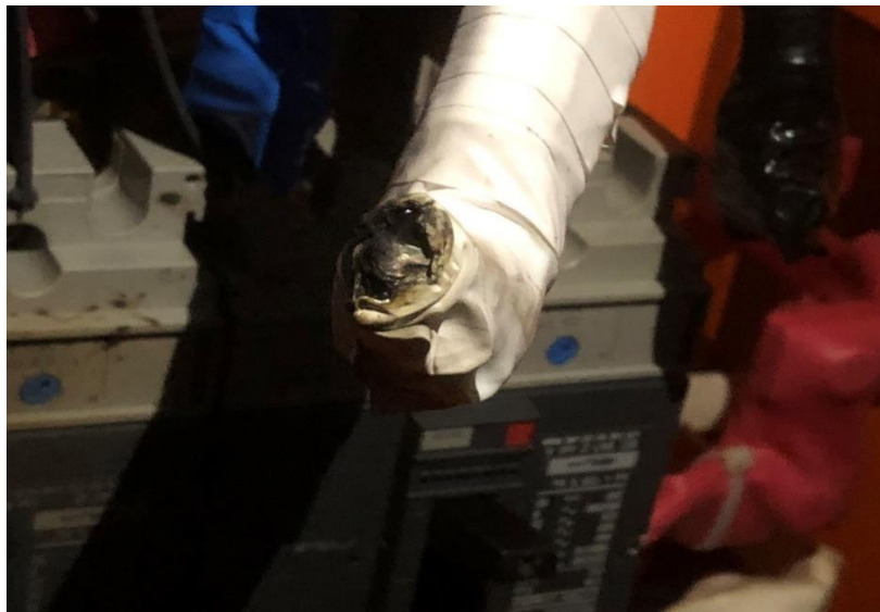
PVC electrical tape used as a temporary insulation over the 'back to back' bolted generator connection.
