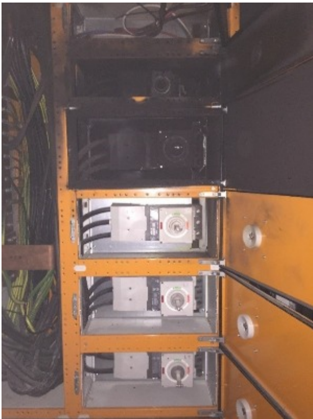
Damage caused by the arc flash explosion.
