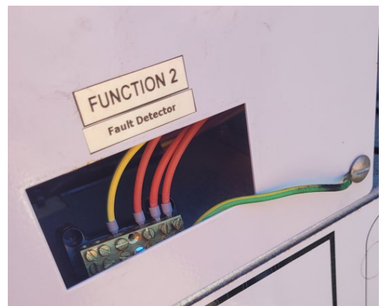
Figure 2: Fault indicator leads shorted and earthed via a terminal neutral link
