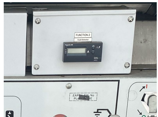
Figure 1: Schneider FLAIR 21D fault passage indicator installed in EFACEC RMU
