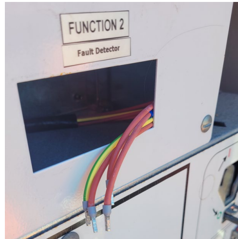
Figure 4: Fault indicator panel with Schneider FLAIR 21D fault indicator missing.
